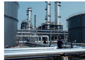
Petroleum and petrochemical
